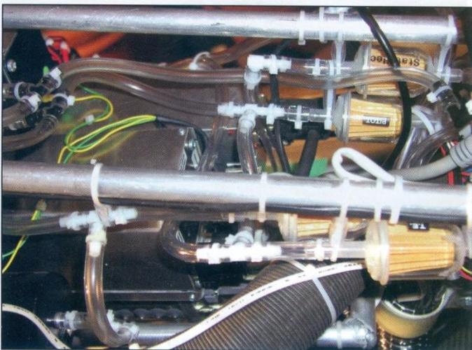
Secured and sealed pneumatic plumbing in the Ventus 2a.
